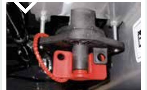
LOG- OUT TAG- OUT BATTERY MASTER SWITCH
